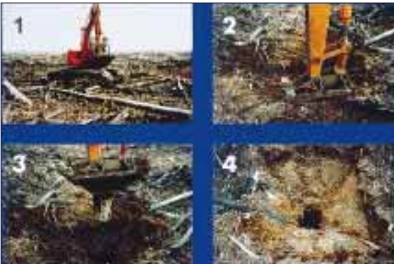
Figure 1. (Clockwise) (1) Excavator with punch attachment, (2) compacting, and (3, 4) preparing a planting hole-in-hole (courtesy of PT Group Plantations, Indonesia).
